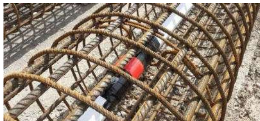
Figure 12 - Monitoring devices installed: inclinometers cases installed inside the bored pile wall.
