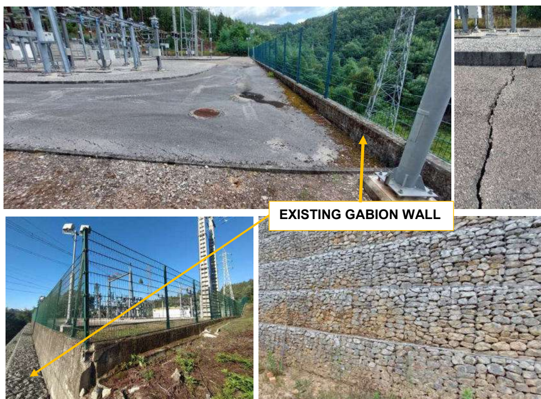
Figure 5 –Existing pathologies in the substation.
