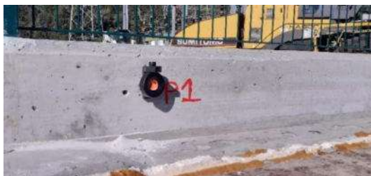
Figure 11 - Monitoring devices installed: topographic prism targets installed in the reinforced concrete wall.
